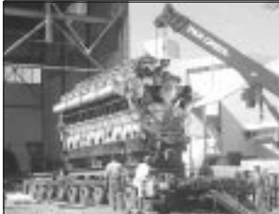
A crane places one of the diesel generators in the old RIF plant of Aqualectra on a special trailer in Curaçao. The 110-ton 16-cylinder Mirrlees Blackstone generators will be taken to the harbour to be shipped out. To remove them, part of the structure had to be saved off. Once all engines have been removed the building will be demolished and the land cleared, so that it can be used for developments related to the megapier for cruise ships nearby.
